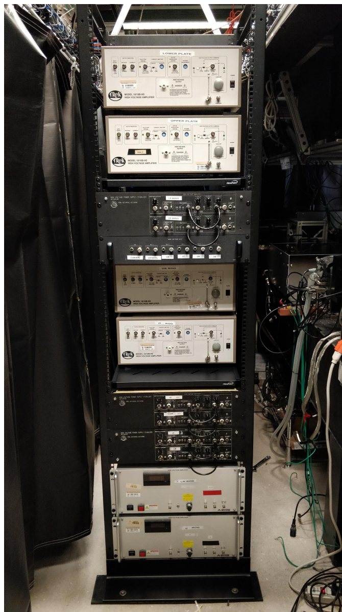
Figure 3.13: High voltage rack holding 6 HV amps, servos, and stable DACs. This picture was taken just after installation of the rack, so many BNC and HV connections are missing.
